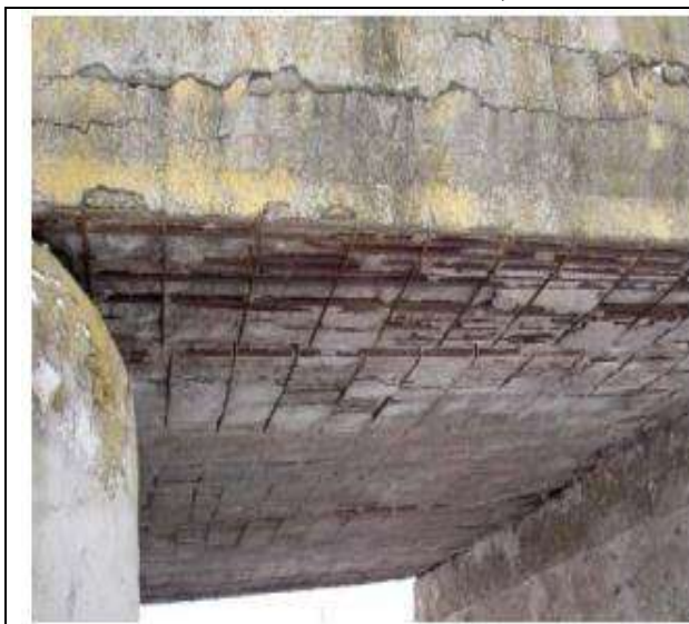
2-rasm. Beton himoya qatlamining to'kilishi
